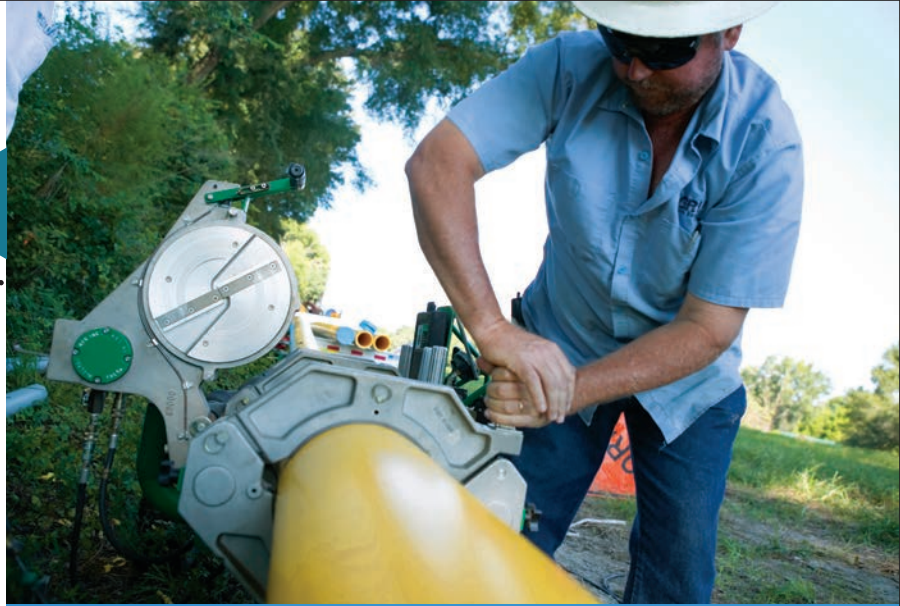
Employees maintain equipment to ensure safety and proper operation while improving reliability.
